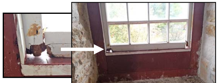
Daylight showing through a rotted out window sash in the Old Stone Mill (close up on left)
