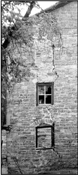
This early 1960s photo of the mill shows one of the many problems, a crack extending almost bottom to top along the south wall of the mill.
